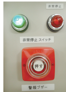
Figure 6-2: Emergency button: in the case of an emergency, accelerator operation can be terminated.
