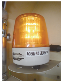
Figure 6-1: Flashing yellow pilot lamp indicates the operation of accelerators.
